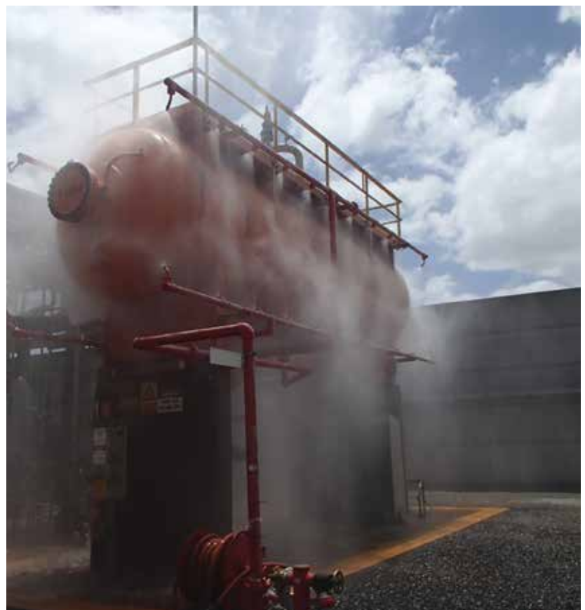
Altona Refinery Deluge System Test
